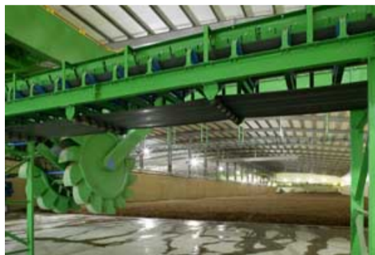
The beam which holds the compost turning wheel in place has broken
